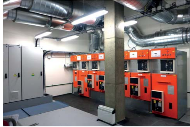
Trafostanice – ON Semiconductor
